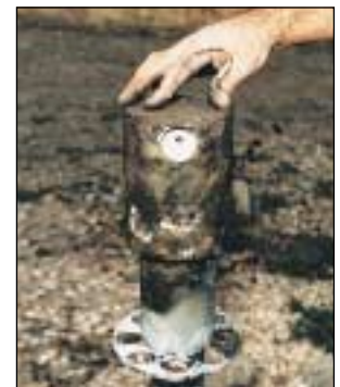
Burned PTFE shows the conductive path formed by dust-laden moisture. As the path arcs over, the transmission line fails.
