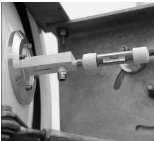
Static Desiccator SD-001 attached to Microwave Antenna Feed.
